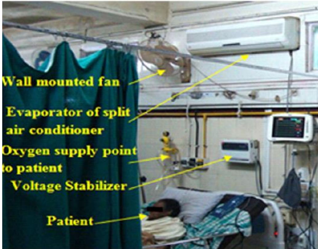
Split air conditioner above the patient's bed in an ICU. Voltage stabilizer is also a potential source
